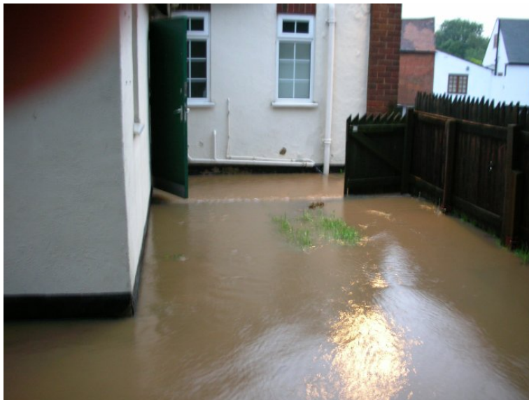
Photo 4 - Village Hall flooding - 2007
